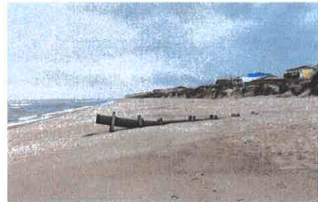
Photo 1: Davis Road Stormwater Outfall During Discharge Event
