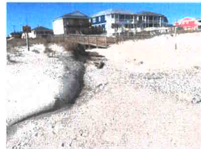
Photo 3: Erosion from overflow area after Hurricane Florence
