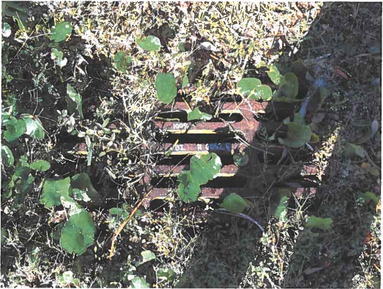
Figure M: Obstructed Inlet Grate
