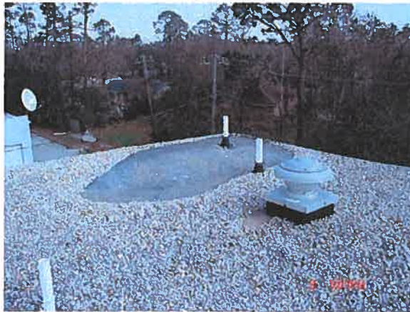
FIG. 5—Wind vortex formation on gravel roofs due to low parapet.
