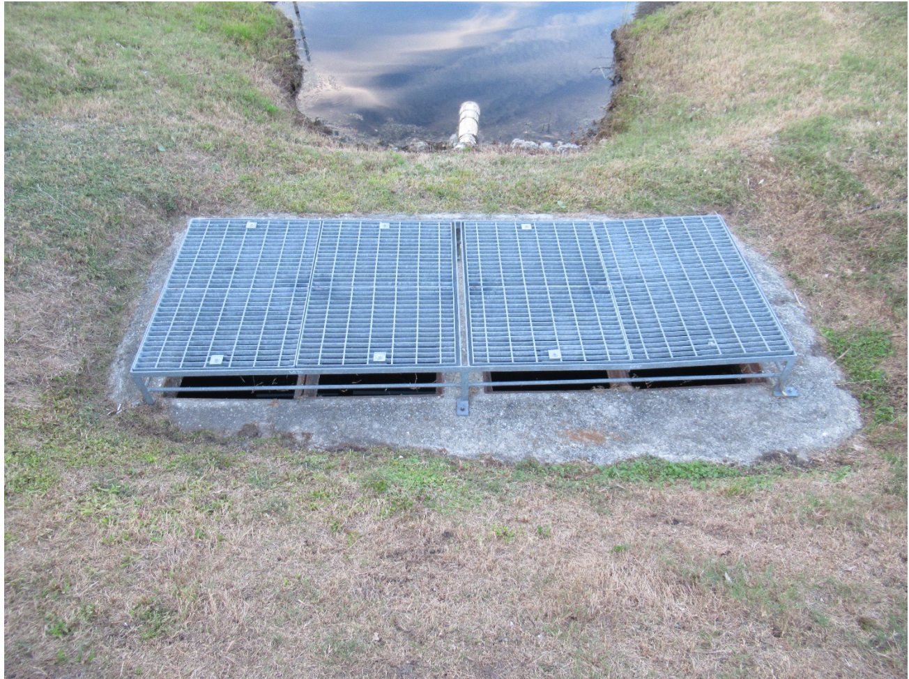
Figure K: Dual Grate Outlet Drain for Pond Network
