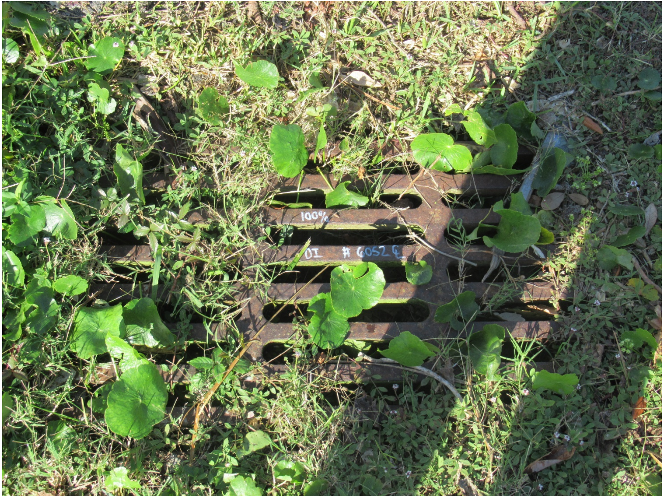
Figure M: Obstructed Inlet Grate
